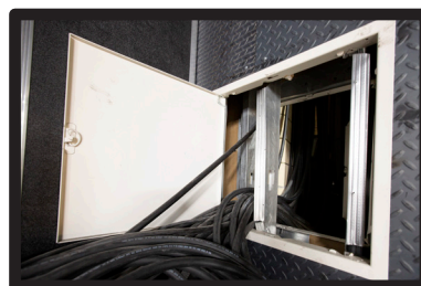
Feeder Pass Through to Electrical Service
